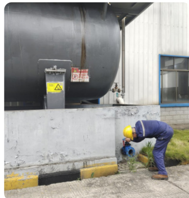
Confirming the emergency collection pool
